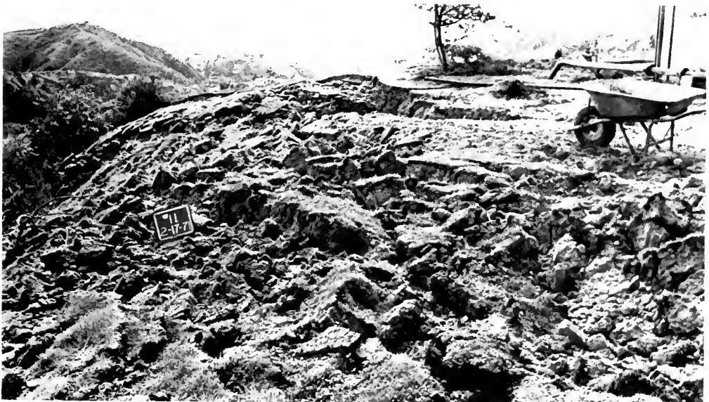
Photo 18. Ground cracks associated with settlement of fill related to consolidation of underlying alluvium and/or slopewash. Courtesy of the Engineering Geology Section, Los Angeles County Engineer's Office.
